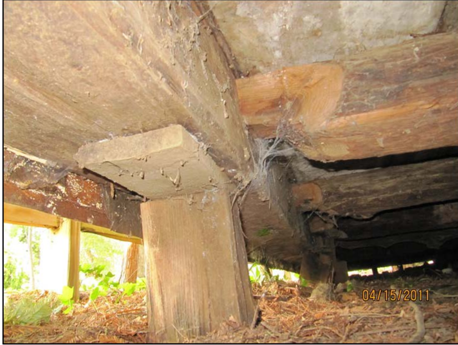
Figure 21. Cunningham House original foundation showing mortise and tenon floor joists, view to southeast, 2011
